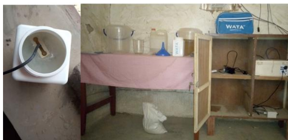
Figure 2 - Photo of an electro-chlorinator device and a production room.
